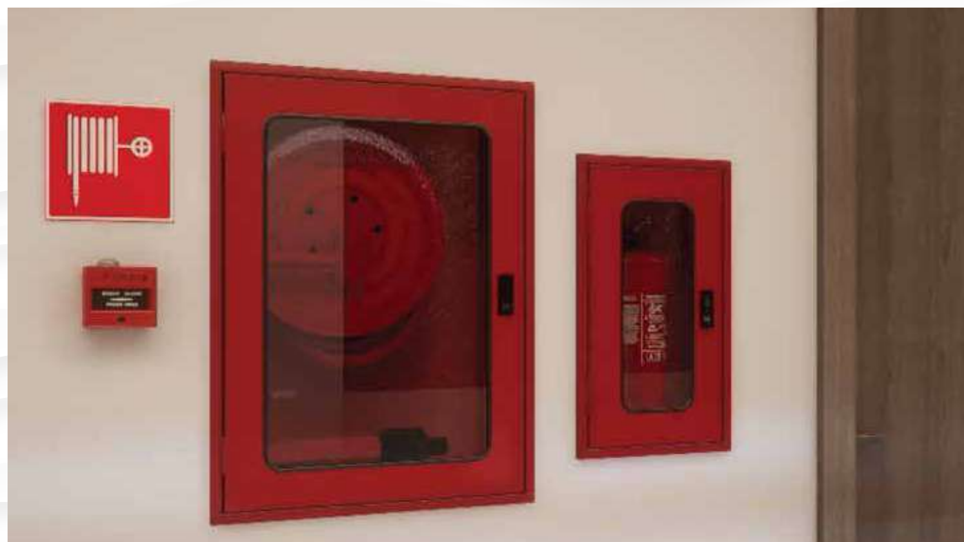
FIRE SAFETY SYSTEM
